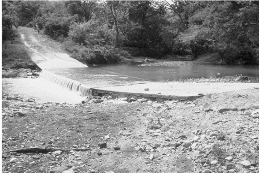
Figure 2.24: A low-water crossing with an armored roadway surface in need of additional downstream scour protection (Keller and Sherar, 2003b)
