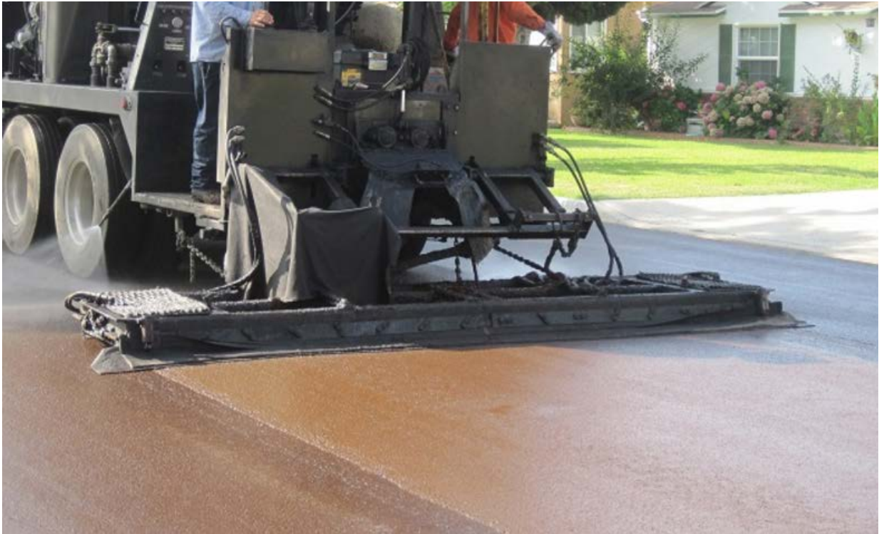
Figure 2.16: Applying and smoothing a Slurry Seal layer on the Surface (LA County, 2017a)
