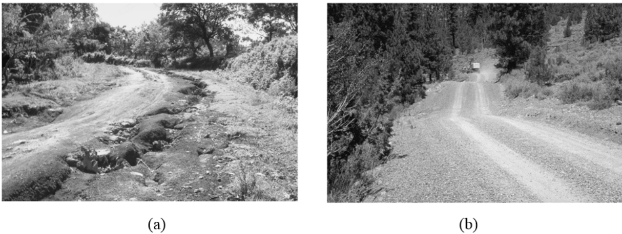
Figure 2.23: The Impact of Drainage Design. (a) A poorly drained road with rutting and erosion problems; (b) An armored road surface with positive surface drainage using rolling dips (Keller and Sherar, 2003b)
